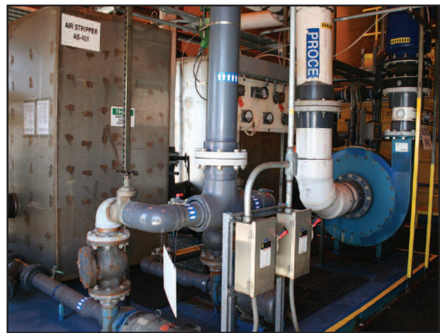
Inside of Water Treatment System
