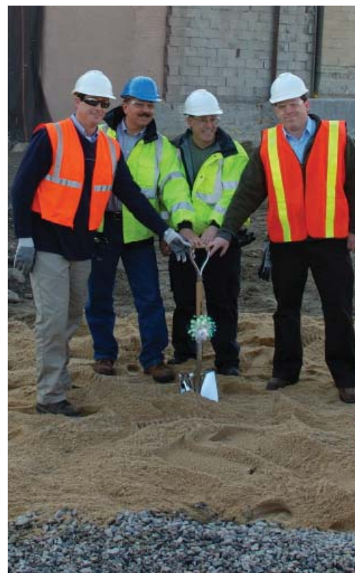
In honor of his 30 years with ExxonMobil, Steve Trifiletti, Greenpoint Remediation Project Manager, broke ground on the new Soil Vapor Treatment facility and office building. Pictured (from left) are members of the Greenpoint Remediation Project team: Justin Kennedy, Steve Trifiletti, Vito Genova, and Chris Proce.
