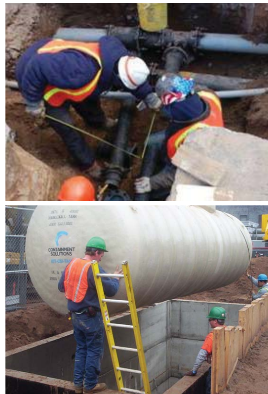
Workers install piping and product storage tanks as part of the 10 new dual-pump recovery wells at ExxonMobil's Greenpoint Remediation Project site. All wells are expected to be fully operational by the end of the year.
